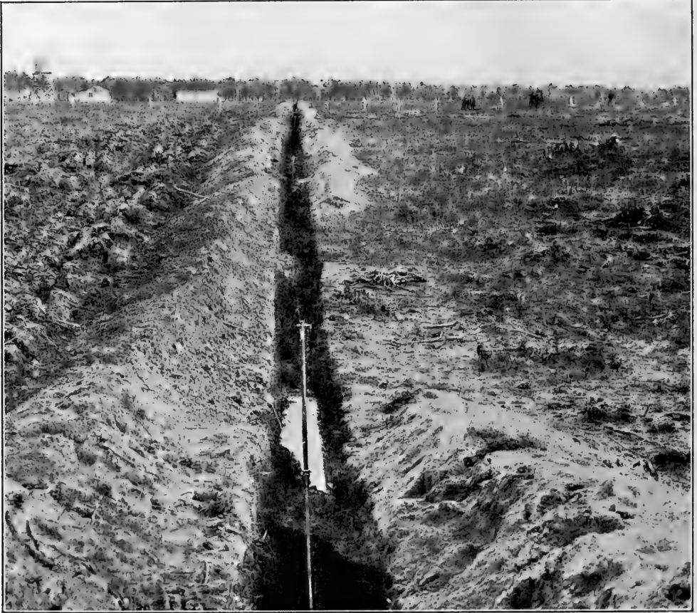
The irrigation trunk line and standards
